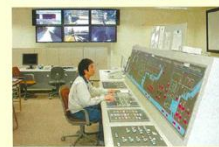
Central monitor and control board of Zempukoji River intake facility
