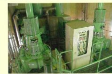
Main discharge pump of Zempukoji River intake facility
