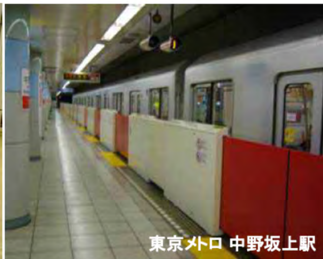
Automatic Platform Gate
